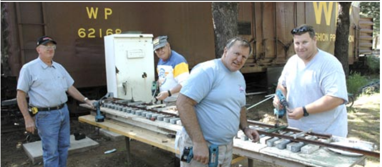
The Track panel gang - Pete Arney, Jack Freedman, Bill Yoder, and Richard Lutrel. They built 18 panels.
