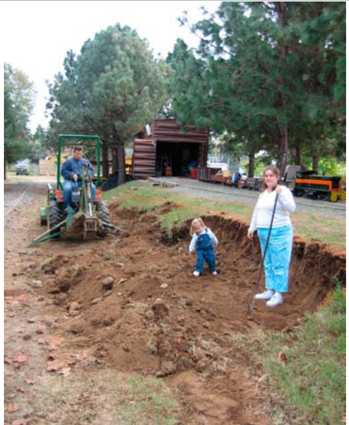
Above: Richard, Amy and Sarah work on digging to make space for container.
