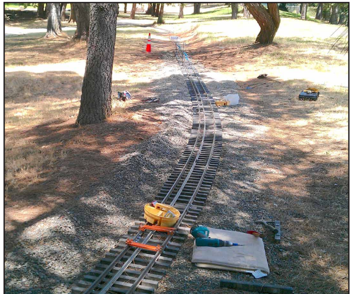
Mainline after realignment. It had been more than a foot to the right of center line.
