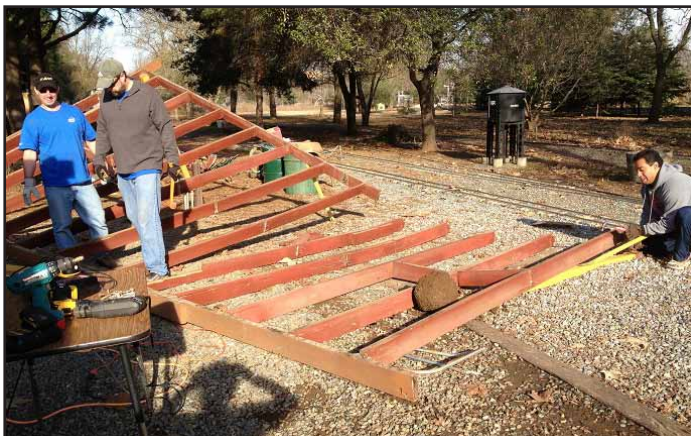
Prior work by Intel crew was to remove the old shade cover, they made quick work. Thanks.
